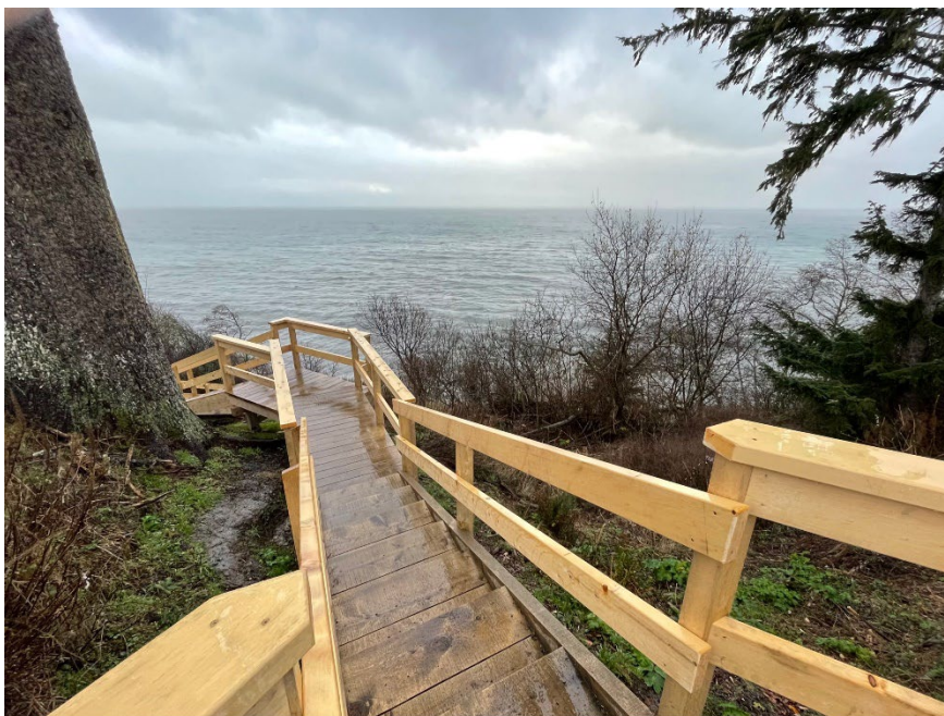
Major repair work completed to the Sooke Bluffs staircase extend the asset's lifespan by 10-15 years.
