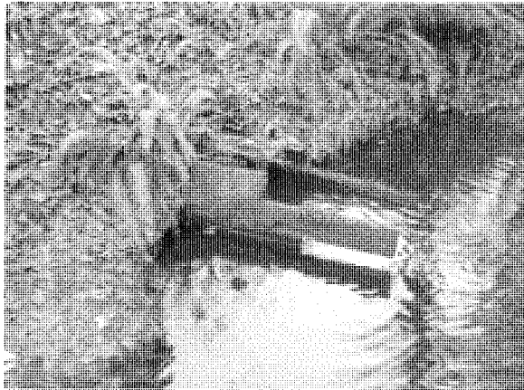
Culvert outlet clearly showing deteriorating conditions
