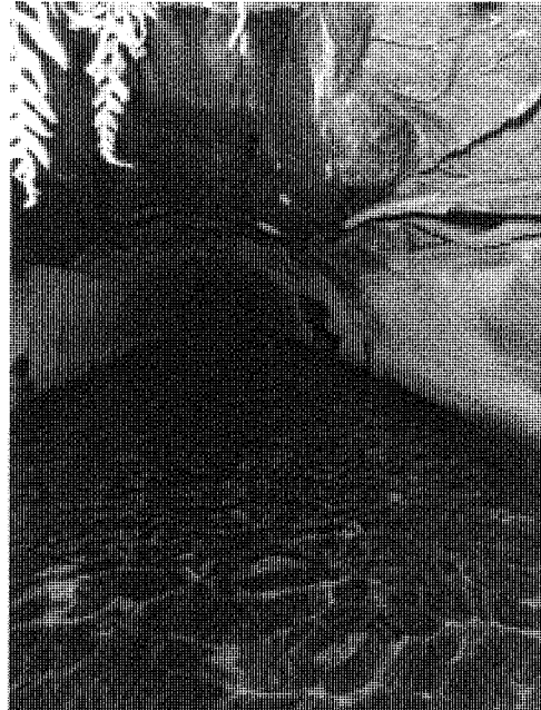
The wood stave has disengaged from the metal support
